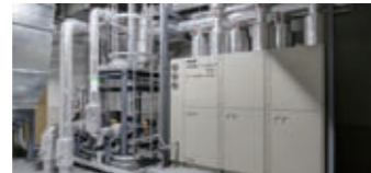
Geothermal heat pump system
